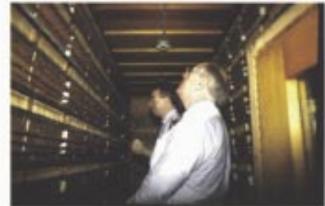
Jack and Doug inside the "keyer" relay in the Right Stage Chamber. This is a smaller, pressurized room, within the actual "relay room".
