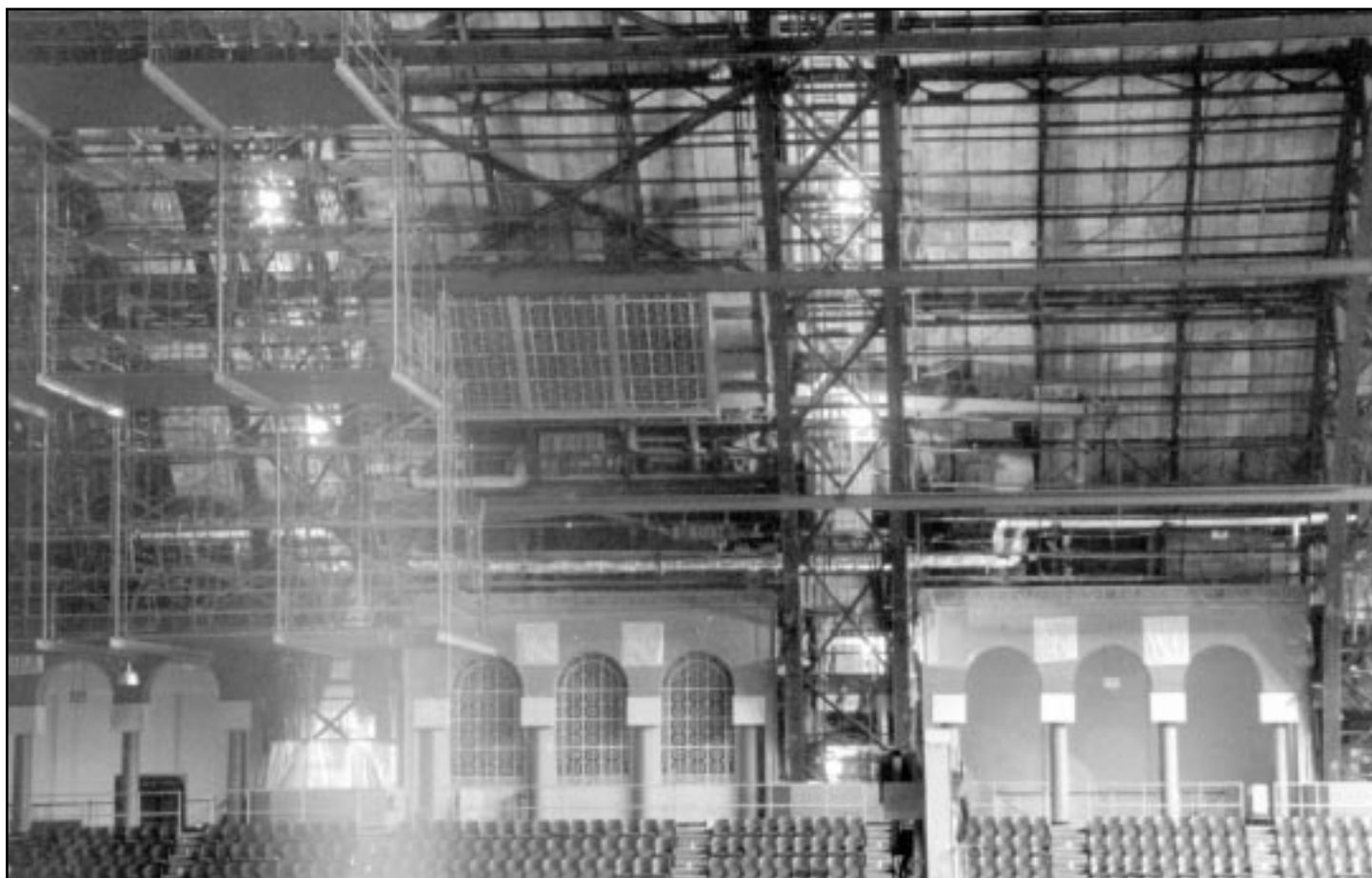
The Fanfare chamber and, to its right, the Trombone seen from the opposite side of the auditorium.
