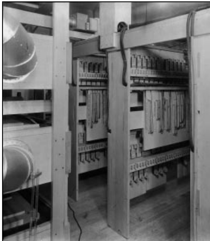
A section of the relays for departments in the Right Stage and R equipment is housed in a room above the entrance to the hall!
