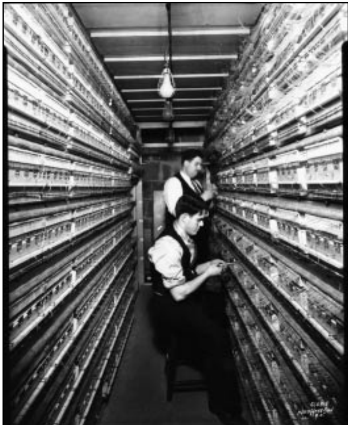
“Keyer” relay room for the Left Stage and Left Forward chambers. This is the nerve center for the Pedal Left, Choir, Unenclosed Choir, Swell, Swell-Choir, and String I departments.
