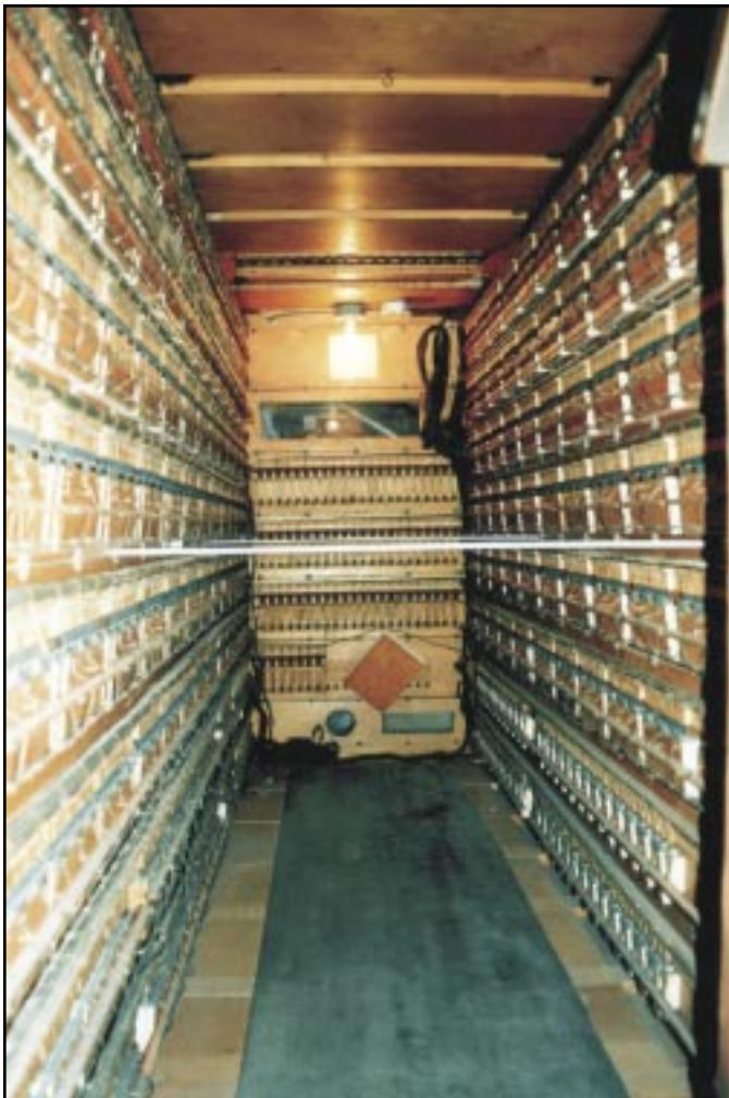
Interior of the "keyer" relay room for the departments sited in the Right Stage and Right Forward chambers.
