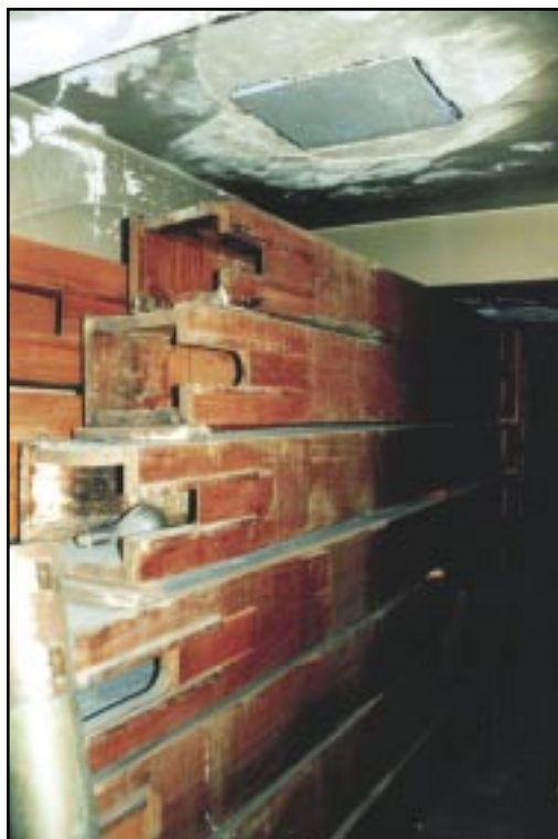
The horizontally-installed basses of the Gallery III organ's Contra Diapason have received a thorough drenching at some stage(s) and the chamber walls, etc., are in a poor condition.
