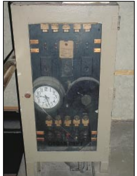
The original blower control panel for the Midmer-Losh organ located on the wall to the left of the kiosk.
