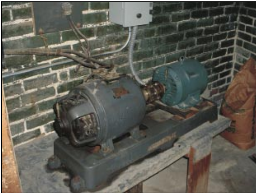
The original DC generator for the Midmer-Losh organ. It is located in the blower room for the Right Stage chamber. The new AC motor was installed about twelve years ago.
