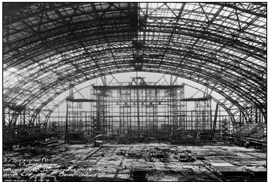
The steel skeleton for Boardwalk Hall takes shape in 1928. The Left and Right Stage chambers will be installed at either end of the stagehouse steel work seen in place. (Photo courtesy of Atlantic City: 125 Years of Ocean Madness by Vicki Gold Levi & Lee Eisenberg)
