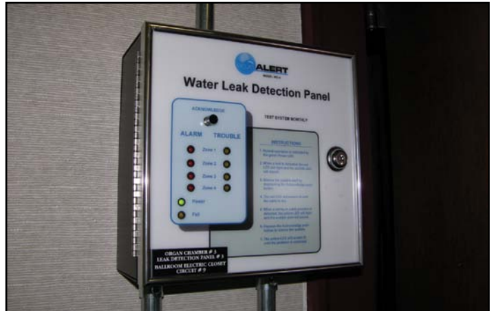
Example of one of the moisture system alarm panels installed throughout both organs in Boardwalk Hall. Photo by Harry Bellangy.
