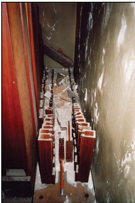
Treble pipes of the Melodia. When workmen gouged a hole in the chamber's wall for a new service pipe (visible in the top left of picture 6), these pipes were covered with plaster and other debris. The same thing has happened in other chambers.
