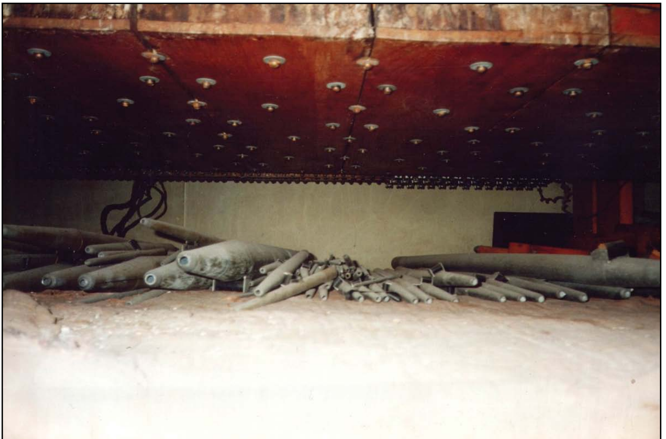
Pipes from some ranks in the String II organ are stored under their water-damaged chests.
