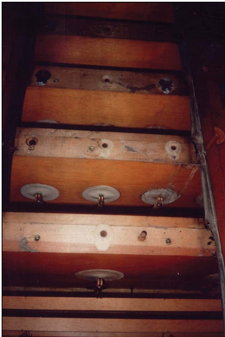
Underside of a chest in the String II organ. Some leathers appear to be in reasonable condition, whilst others have obviously been affected by water.
