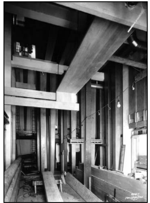
At floor level in the Right Stage chamber. Gradually, more and more of the 64-foot stop's pipes are built and maneuvered into position, but they are still without their boots. On the right (aligned with the light bulb) is the CCCCC# pipe, with CCCCC next to it. Arrayed across the picture (left to right) are the pipes for notes GGGGG# down to DDDDD (the latter being positioned next to CCCCC).
